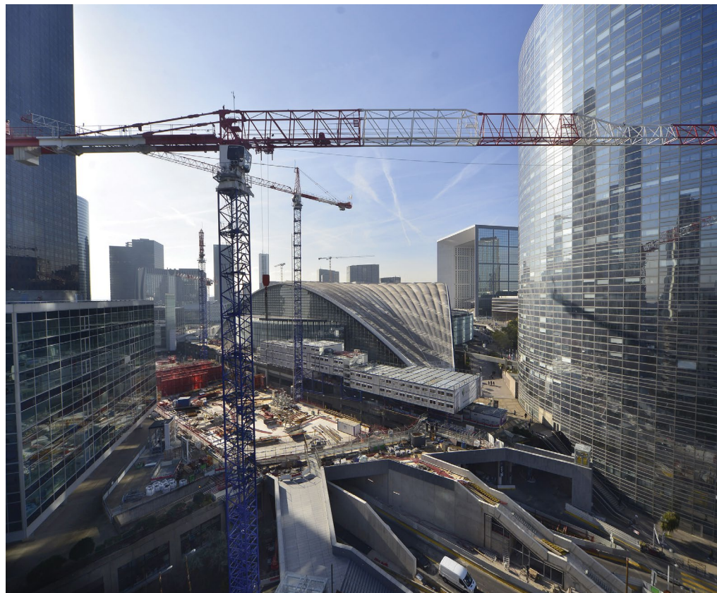
Figure 5. While the tower was under construction, the highway was kept open at all times. © Laurent Zylberman
